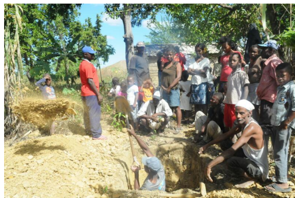
Figure 6. Neighbors helping each other to dig pits in preparation of building their own latrines
