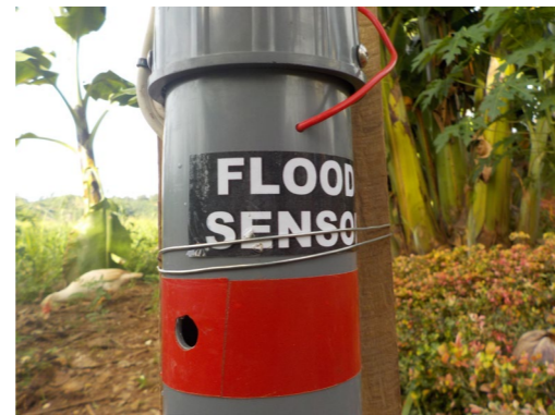
Flood sensors installed near communities prone to flooding
